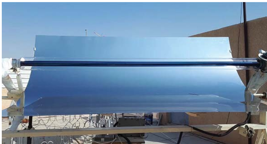
Fig. 3. Parabolic Solar Collector
