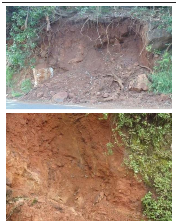
Fig. 1: Land slip occurred during the site visit
