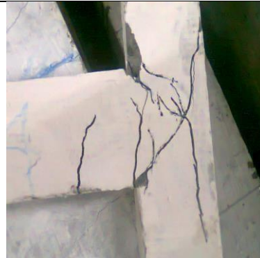
Fig. 8(b) Failure pattern of TS-A
