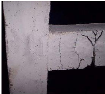
Fig.8(c) Failure pattern of TS-B
